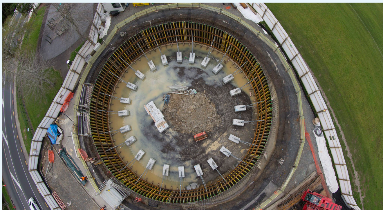
Harold Moody tank: The new structure being constructed in the carpark will be sunk in a controlled exercise.
